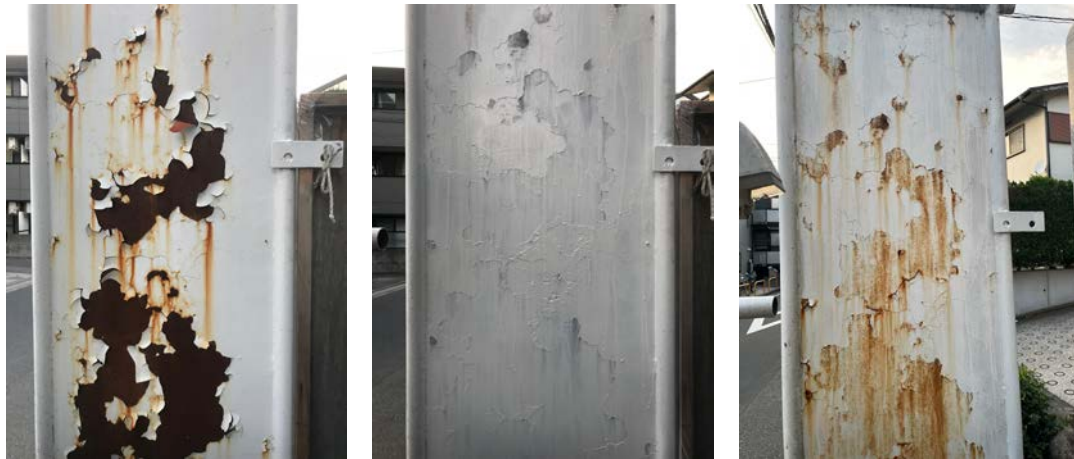
(a) Weathered coated plate (October 30, 2018)
