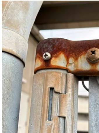
Fig. 9.16 Snapshot of actual galvanic corrosion. The screw has a lower ionization tendency than the body, so it retains its metallic luster, but the body corrosion is accelerated near the screw
