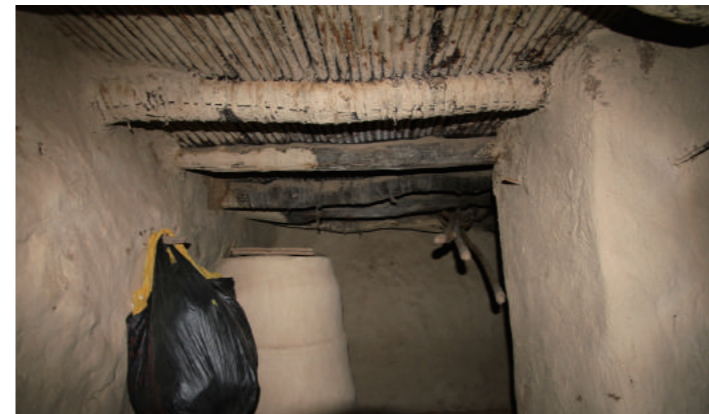
[6] Detail of a Slab between Ground Floor and Upper Floor, photo by Shimizu, N., 2015
