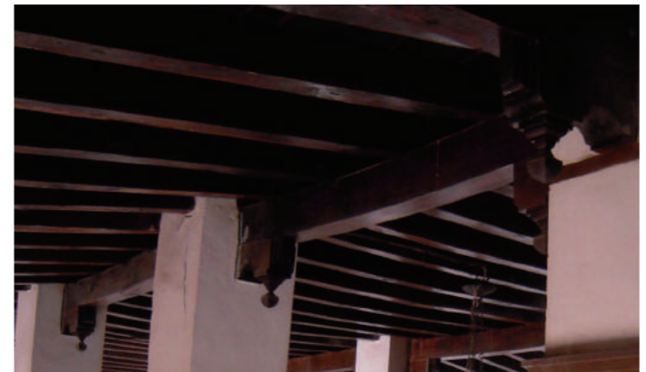
[10] Masonry Pillars with Timber Ornament and Timber Ceiling (Ground Floor, Building-A); Photo by Smidt, W., 2010
