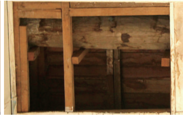
Fig.4-114 The slab structure composed by timber members (photo taken from the ground floor), Liquor Factory, photo by author.
