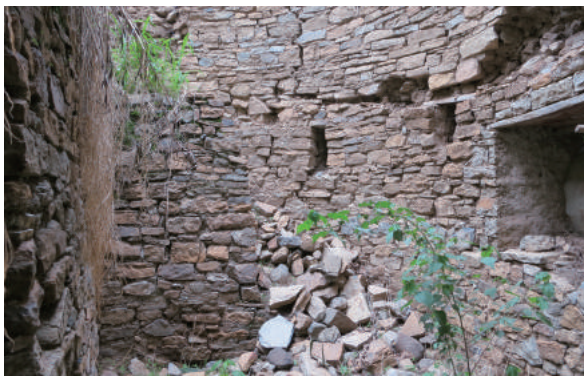
Fig.4-104 Presently ruined stairs, Building-B of Gugsa's Second House, photo by author.
