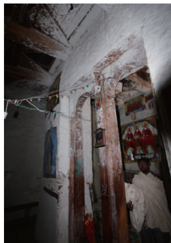
Fig.2-105 Timber screen between pillars, which separates qiddist from qiné mahlét , Debre Sillasé Church, photo by author.
