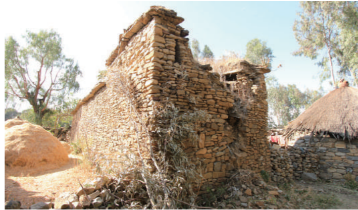
[2] A Collapsed Wall in the Eastside, photo by Shimizu, N., 2015
