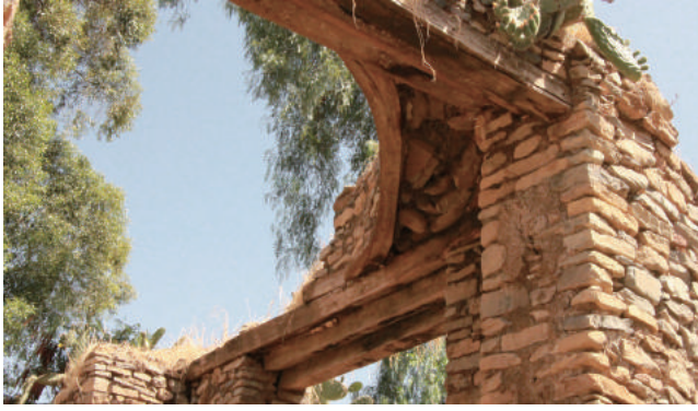
Fig.4-16 A rectangular shaped core switched to a cylindrical shape in the upper part, Residence of Ras Welde Sillasé in Ch'eleqot, photo by author .
