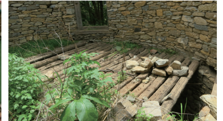
[9] Upper Floor of the Building-B Floored with Timber Members, photo by Shimizu, N., 2012
