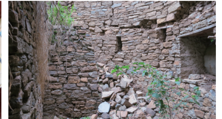
[11] Collapsed Stairs and Cracked Masonry Wall (building-B), photo by Shimizu, N., 2012
