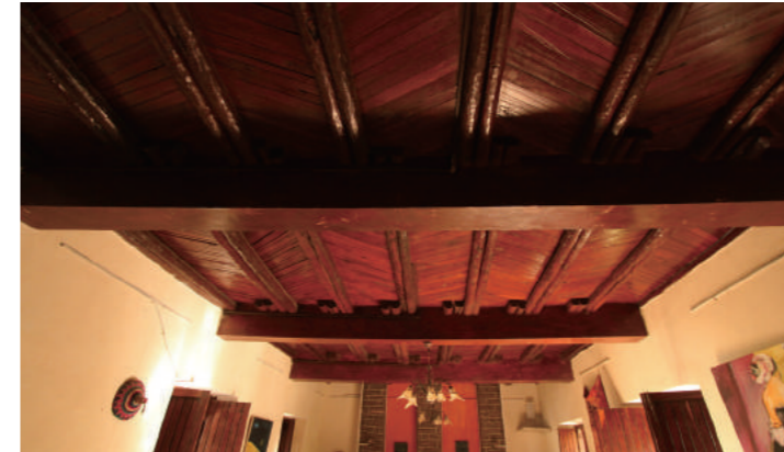
[8] Hidmo-inspired Timber Ceiling (Perhaps Beam is with RC member), photo by Shimizu, N., 2016
