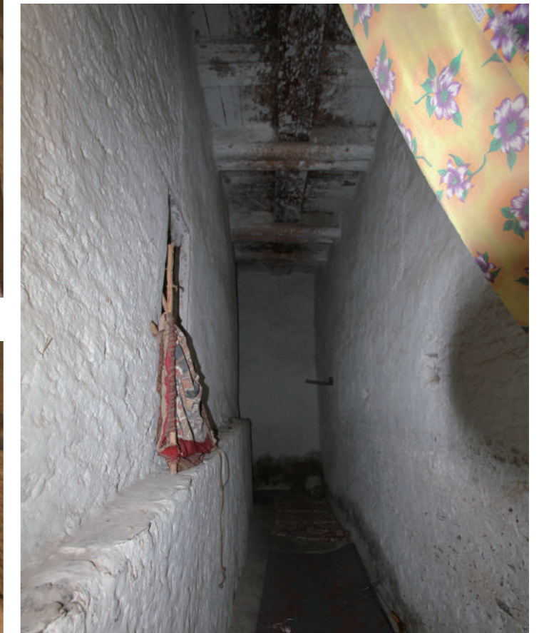
[10] Internal Appearance of Corridor between Meqdes and Eastern Wall, photo by Shimizu, N., 2018
