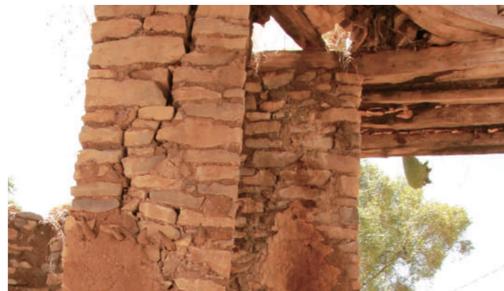
[5] Detail of Cracked Masonry Work with Horn, Photo by Shimizu, N., 2013
