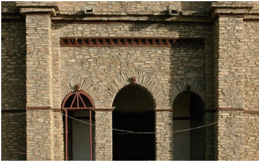
Fig.4-50 Arches installed in the entrance, main building of Emperor Yohannis IV Palace (shortly before the restoration), collection of IPHC.
