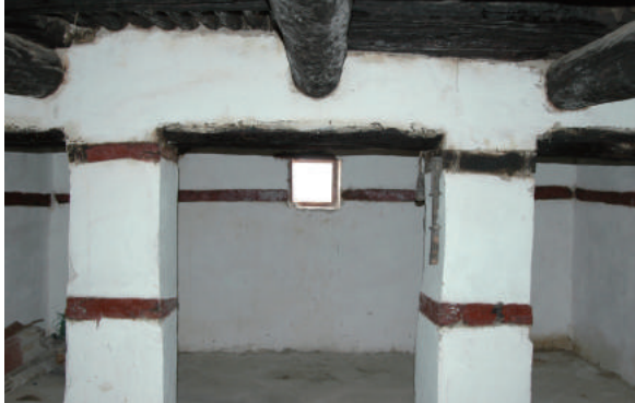
Fig.4-37 Internal appearance of ground floor, Former Residence of Emperor Yohannis IV (Building-B), photo by Mano, Y.
