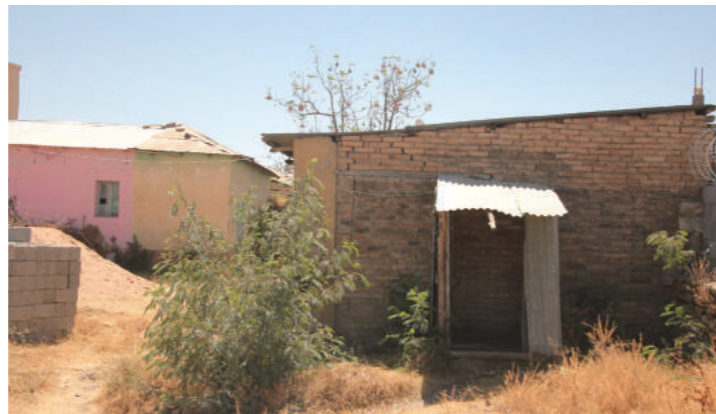
[19] Brick-used Northside Wall of Building-C (from the North); photo by Shimizu, N., 2018
