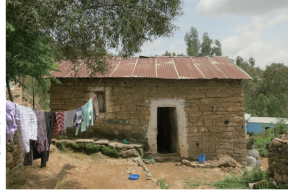
Fig.3-65 An example that local hidmo ceiling and roof were replaced by corrugated metal sheet. photo by author.
