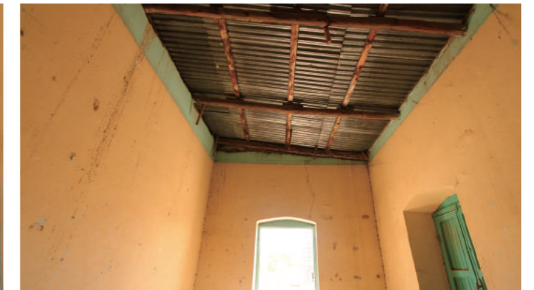
[10] Roofing Structure Exposed by Ceiling Unfastened (Upper Floor, B-Part), photo by Shimizu, N., 2016
