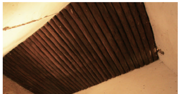
Fig.4-23 Ceiling simply consisting of row of timbers, Ar'aya Castle, photo by author.
