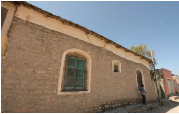
Fig.4-176 External appearance from the street, a house nearby Liquor Factory, photo by author.
