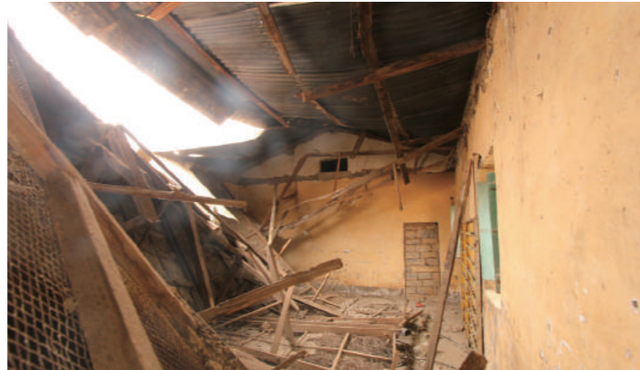
[15] A Collapsed Situation before Reinforcement, photo by Shimizu, N., 2016
