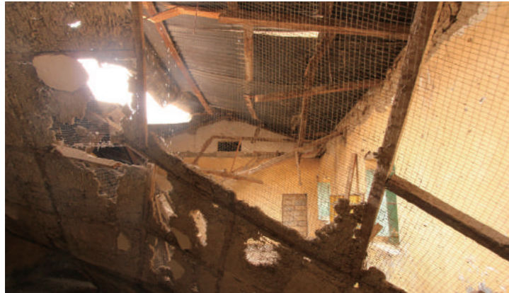
[14] A Collapsed Situation before Reinforcement, photo by Shimizu, N., 2016
