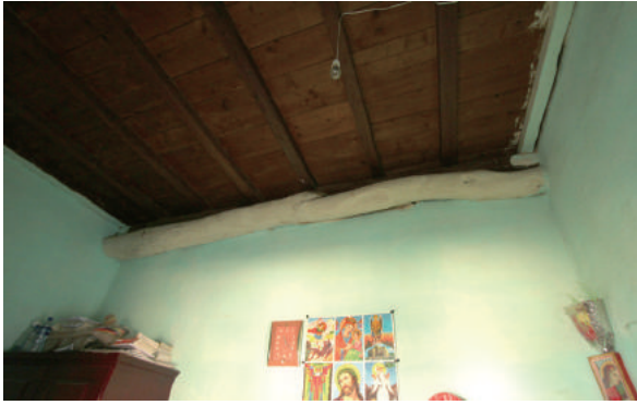
Fig.4-148 Ceiling of ground floor, Building-A of Old Hospital Quarter, photo by author.
