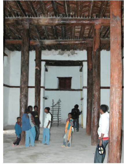
Fig.4-31 Internal appearance after restoration, Former Residence of Emperor Yohannis IV (Building-A), photo by Mano, Y.
