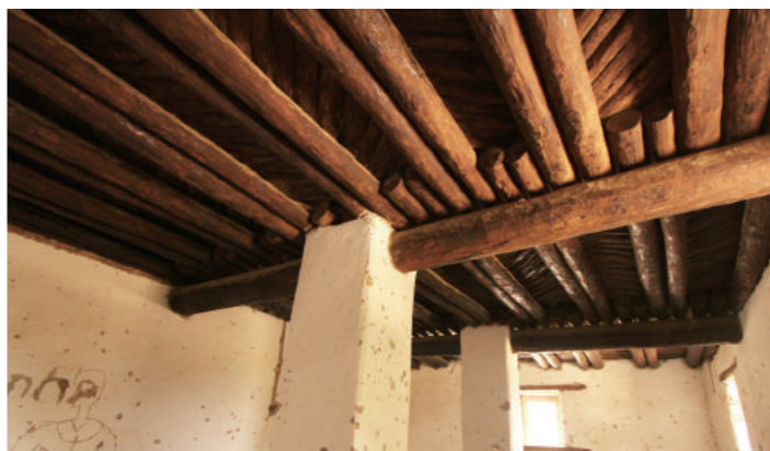
[12] Masonry Pillars and Wooden Ceiling of a Room on the West Side in the Ground Floor, photo by Shimizu, N., 2018
