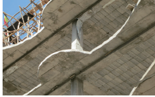
Fig.4-199 A building that material of a concrete block is applied in slab, photo by author .
