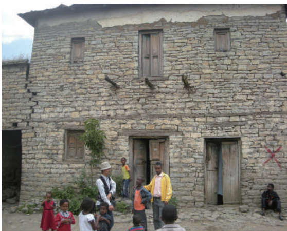
Fig.4-69 An example of a two-story house with symmetric facade. The marking of "X" found in lower right means that demolition is planned, photo by author .
