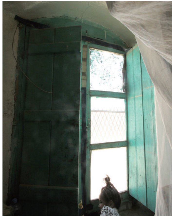
[6] A Timber Window in Arched Shape Masonry Wall, photo by Shimizu, N., 2016
