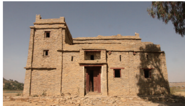
[5] Present State after the Collapse of Several Parts of Masonry Wall and Coronal-shaped Ornaments (from the East), photo by Shimizu, N., 2018
