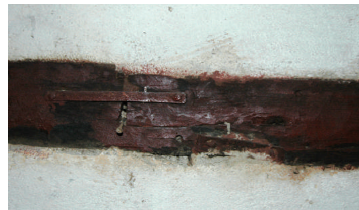
[11] Jointed Part of Timbers Braced by Clamp (Date of Installing Clamp Unknown), photo by Mano, Y., 2011
