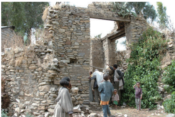
Fig.4-13 A circular and ruinous building for Ras Welde Sillasé in Ch'eleqot, photo by Mano, Y.
