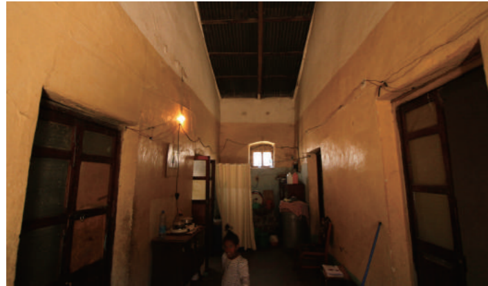
[3] Internal Appearance of a Central Room with Corrugated Metal Sheet Roof, photo by Shimizu, N., 2016
