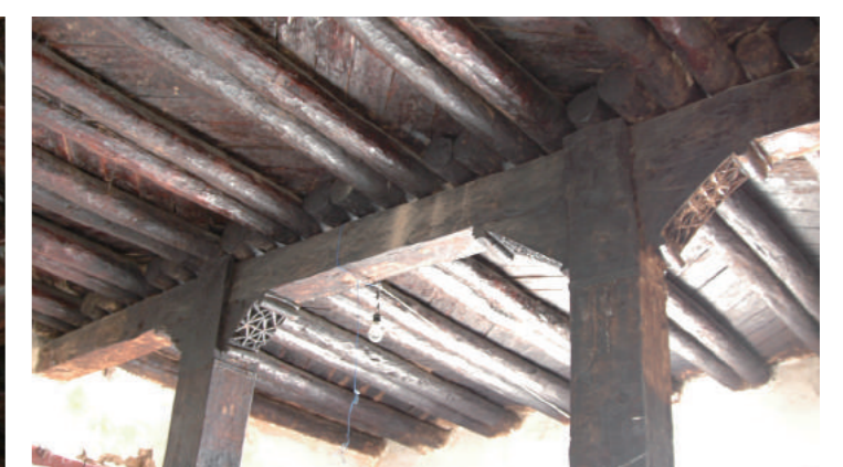
[10] Timber Ornamental Pillars and Ceiling of Building-B (Upper Floor; in Common with Hidmo), photo by Mano, Y., 2011
