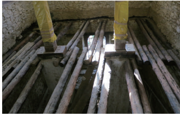
Fig.4-61 Masonry pillars (ground floor) and timber pillars (upper floor) during restoration, residential building of Emperor Yohannis IV Palace, photo by author.
