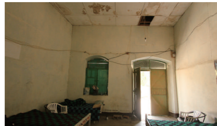
[12] A Room with Panel Ceiling in the Ground Floor of B-Part, photo by Shimizu, N., 2016
