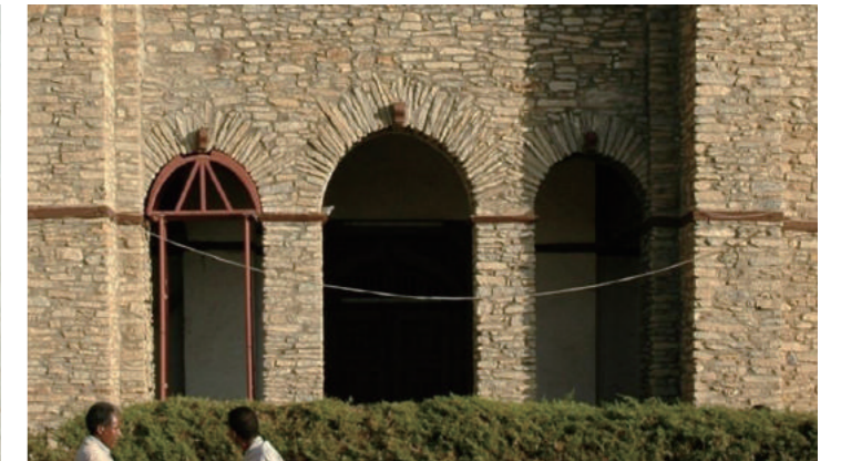
[7] Masonry Arches at the Entrance (Building-A, Shortly Before the Restoration); Collection of IPHC
