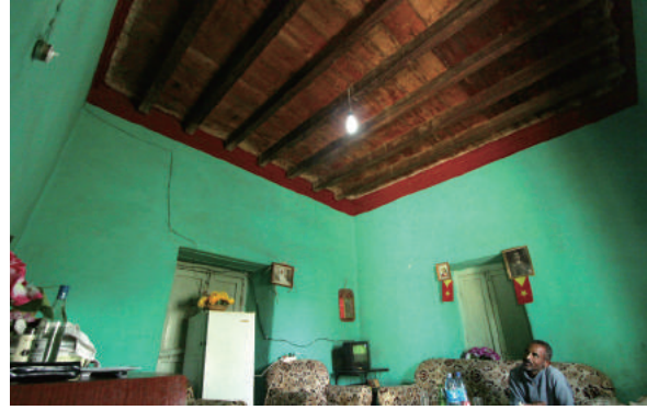
Fig.4-123 Ceiling of ground floor of an example of a two-story house with symmetric façade (Fig.4-71, 122), photo by author.
