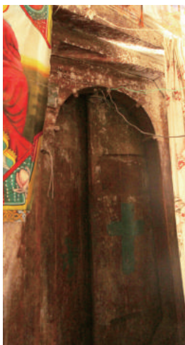
Fig.2-104 A door installed in the west wall of meqdes , Debre Sillasé Church, photo by author.
