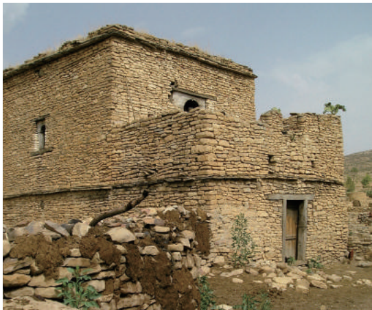
Fig.4-39 External appearance before restoration, Former Residence of Emperor Yohannis IV (Building-B), photo by Smidt, W.
