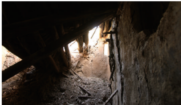
[6] Upper Floor in a State of Collapse, photo by Shimizu, N., 2015
