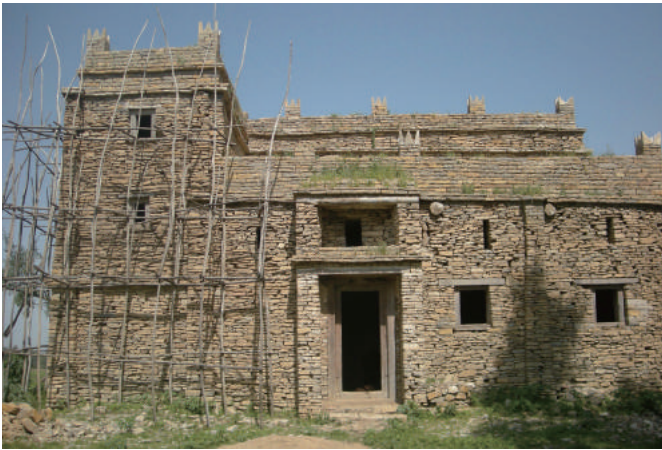
Fig.4-26 External appearance from the east before maintenance, Ar'aya Castle, photo by author.
