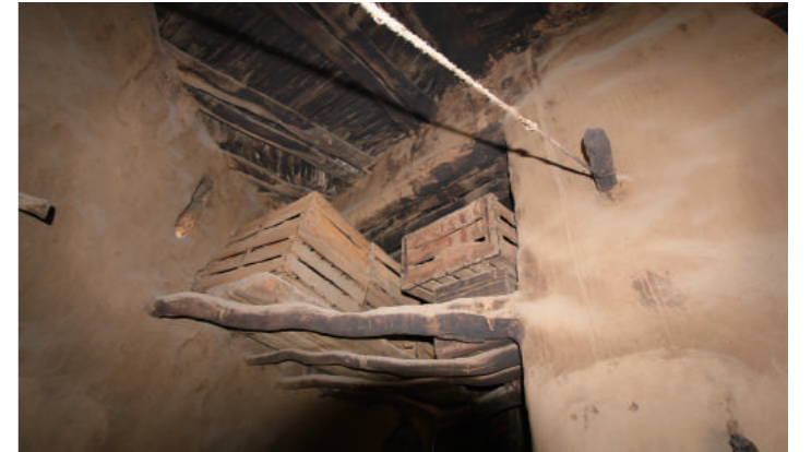
[4] A Central Masonry Pillar and A Built-in Rack, photo by Shimizu, N., 2015
