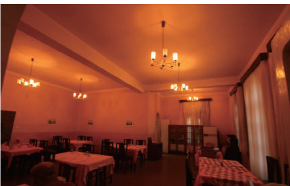
Fig.4-186 Ceiling with RC beam in the ground floor, Abriha Castle, photo by author.
