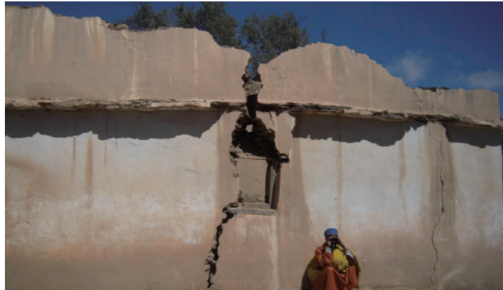
[13] Heavy Crack in the South Wall, photo by Miyake, R., 2009
