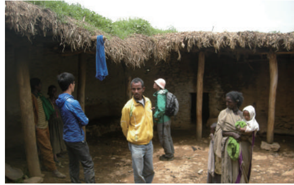
Fig.3-33 Rectilinear courtyard with a roof in a parcel in 'Agame, photo by author.
