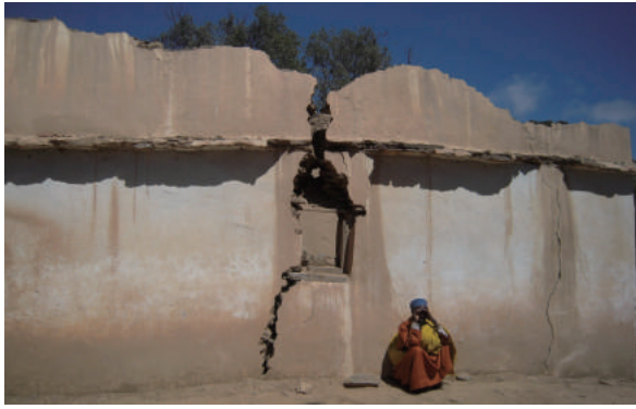
Fig.2-87 Serious crack in the south wall, old church of Asir Metira Monastery, photo by Miyake, R. (taken before the demolition of meqdes).
