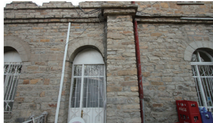
[7] Different Type of Masonry Works between Original Part (Right) and Extended Part (Left), Photo by Shimizu, N., 2018
