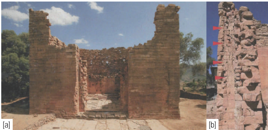
Fig.2-18 Great Temple of Yeha (a: External appearance; b: Wall from a side), from ARCCH et al.
