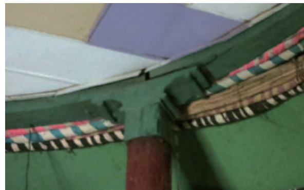
Fig.4-102A timber pillar with bracket capital, Building-A of Gugsa's Second House, photo by author.
