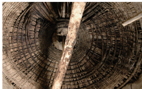
Fig.4-5 A beam bridging over the rectangular core and a king post, photo by Mano, Y.
