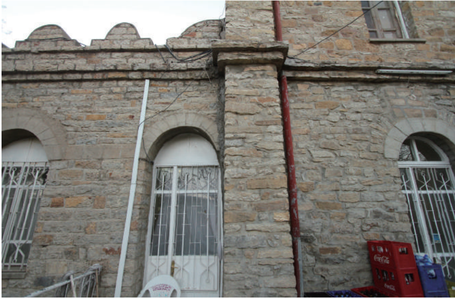
Fig.4-183 Different masonry works between original part (right) and extension part (left), Abriha Castle, photo by author.
