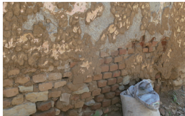
Fig.4-159 A building located in Kwiha that bricks are partly applied, photo by author .
