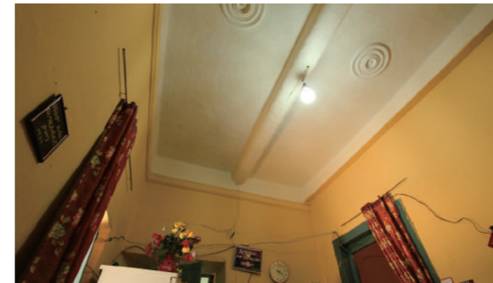
[8] Internal Appearance of a Ground Floor Room on the South Side (Building-A), with a Timber Beam and Plastered Ceiling, photo by Shimizu, N., 2018
