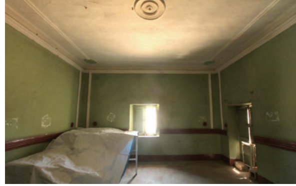
Fig.4-149 Molded ceiling of upper floor, Building-A of Old Hospital Quarter, photo by author.
