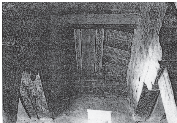
Fig.2-68 Wooden prototype of ridged roof found in the porch of Debre Me'ar, from Buxton (1974).
