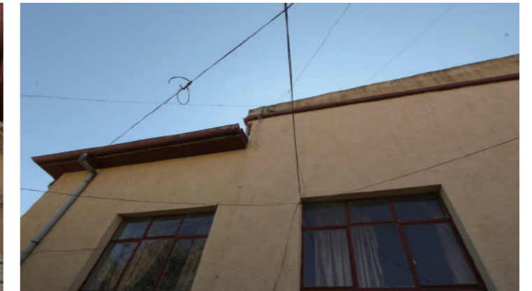
[7] Height of Backside Roof is Lower, photo by Shimizu, N., 2015
