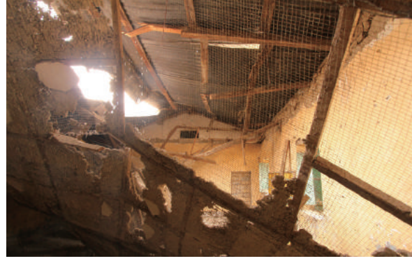
Fig.4-153 A collapsed situation of Building-B before reinforcement, Old Hospital Quarter, photo by author.
