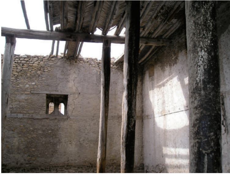
Fig.4-30 Internal appearance before restoration, Former Residence of Emperor Yohannis IV (Building-A) , photo by Smidt, W.
