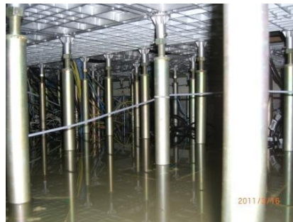
(Flooding inside free access floor of government building <provided by Ishinomaki>)
