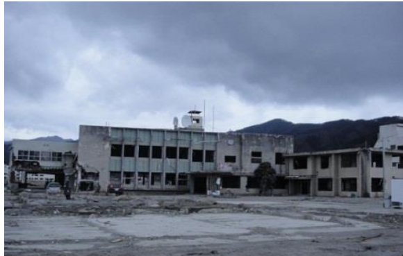
(Damaged Otsuchi town hall and government office building, photographed by author in December 2011)
