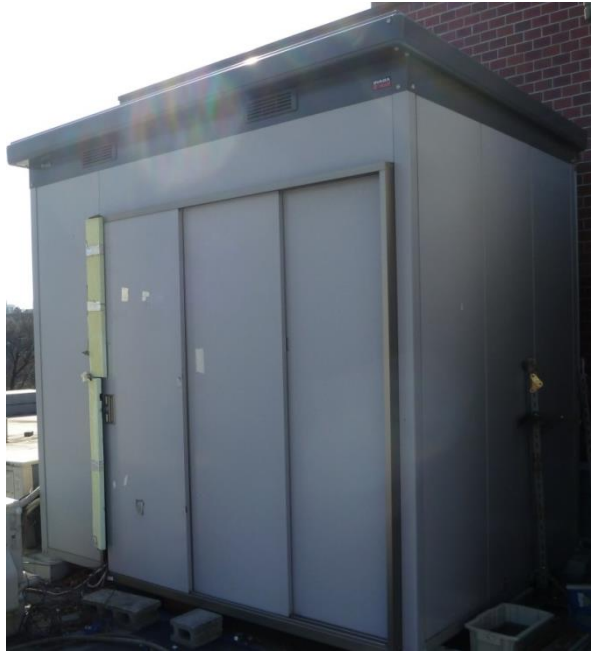
Fig. 14 Air conditioning room for experiment
