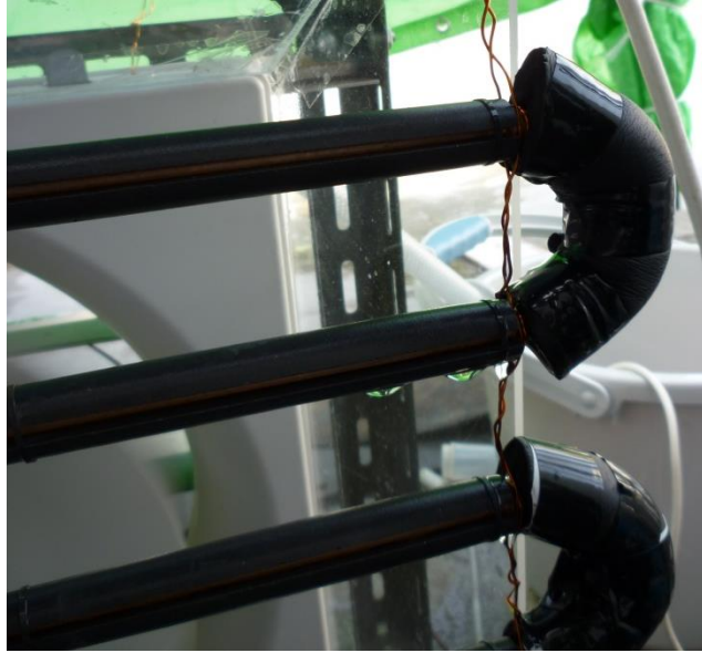
Fig. 19 End of heat exchanger is insulated
