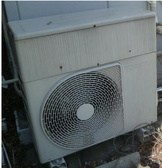
Fig. 26 Outdoor unit of “water” air-conditioning system
