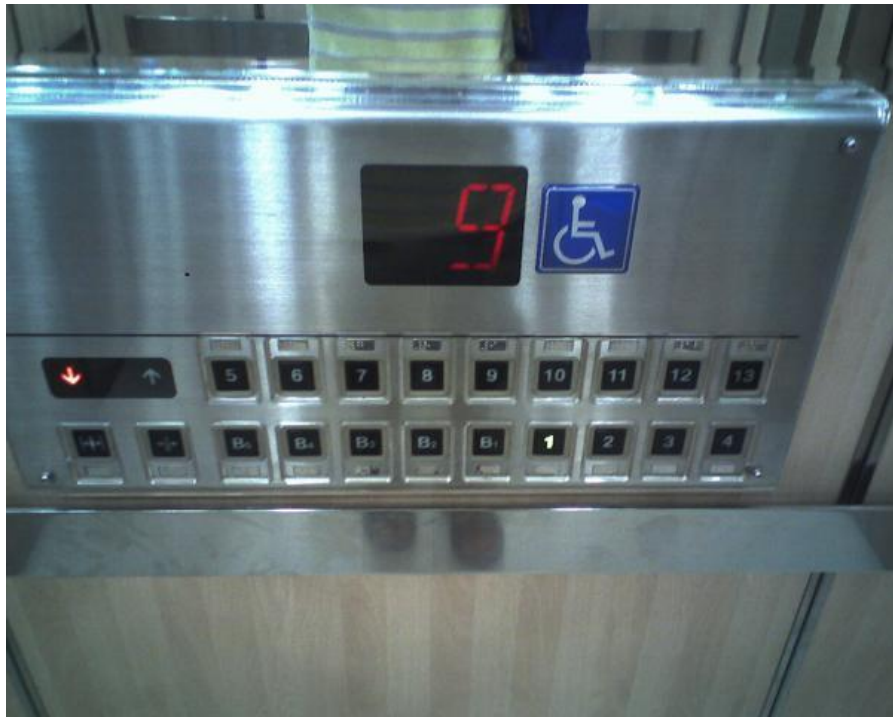
Figure 9: A Handicapped Panel in Elevator
