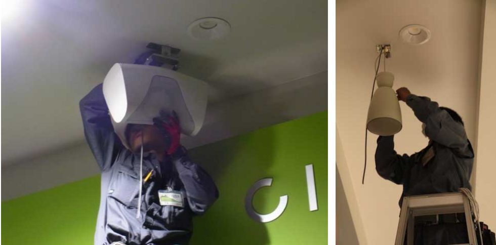
Figure A.22: Putting Speakers in Ceiling
