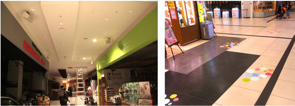
Figure 3.22: Speakers, Step Signs, and Sensors embedded
